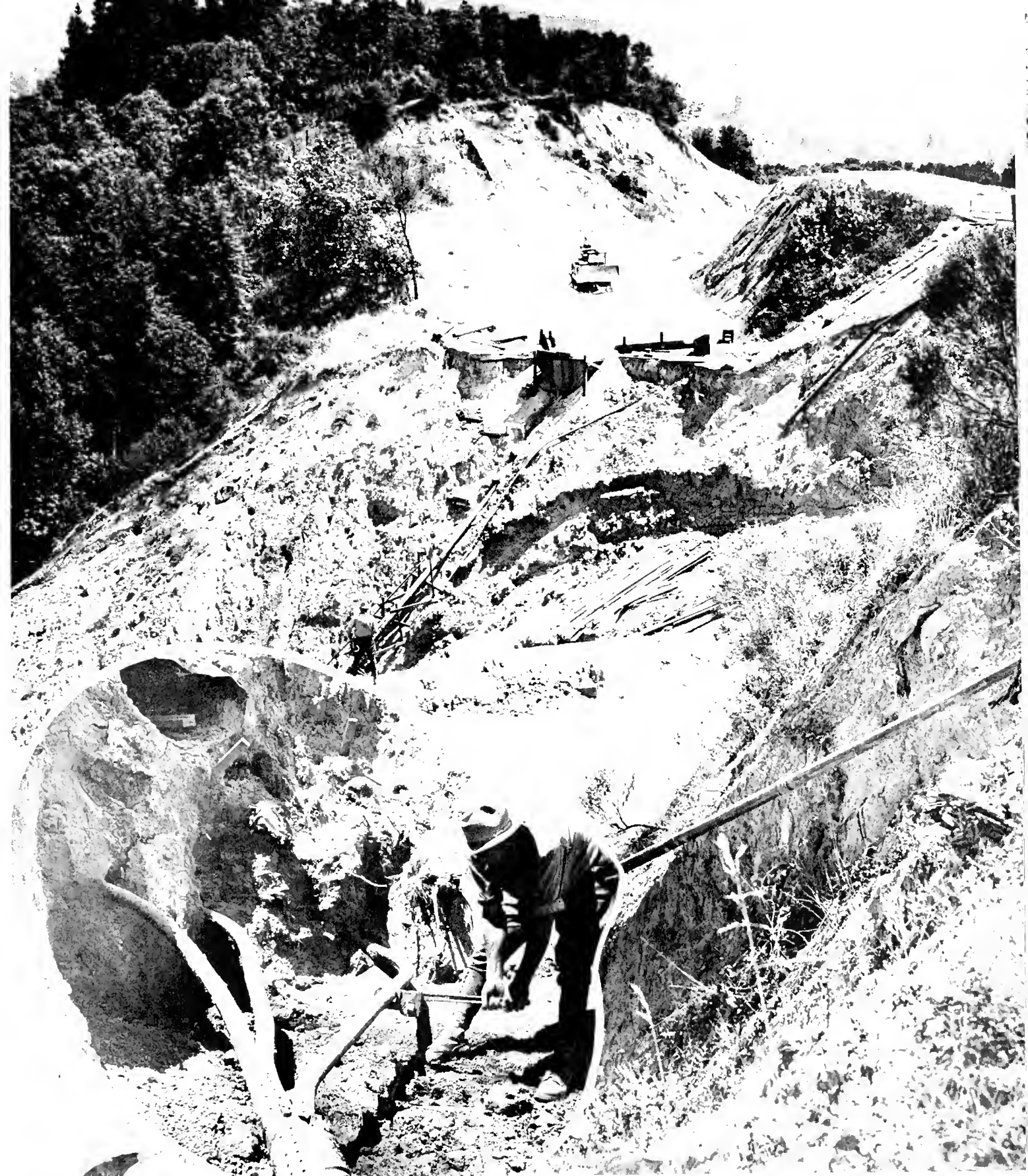
View of large slipout of fill. Installation of extensive drainage system under way. Inset shows outlets of 2-inch perforated pipe drains before covering with crushed rock.
